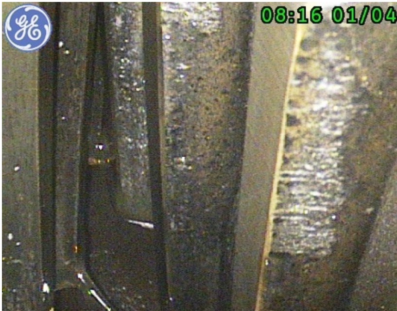
Video Scope Photo. Note concentrated loading on one side of the gear teeth. Indicates a misalignment condition.
